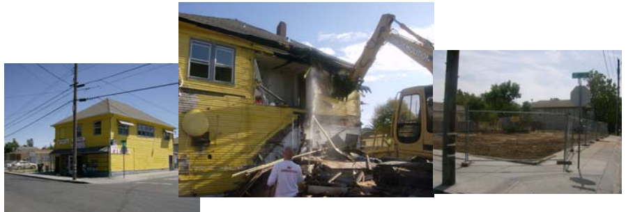
Demolishing the Jay & Gee Market in Oak Park. A single family home will be constructed in its place in 2010.
